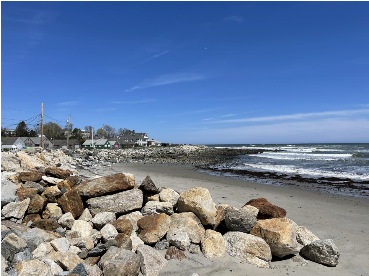
Figure 1. An example of coastal bluff erosion that has since been armored. Historical coastal bluff erosion has destroyed homes, roads, and other resources in this area. The example is from the shore of North Hampton, New Hampshire, and there are several similar sites throughout New England.
