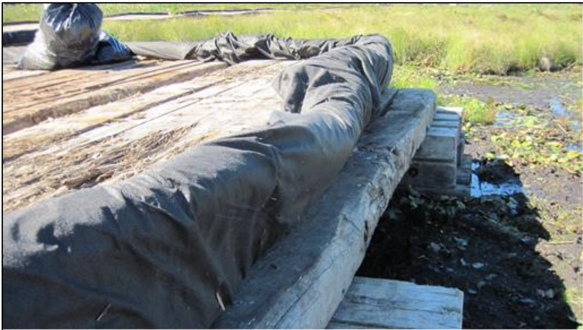
Constructing a swamp mat bridge span reduces direct impacts to the wetland surface and maintains aquatic organism passage through the construction area. The number of necessary swamp mats may be reduced using this method.
