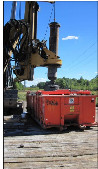
Auger dredge material stockpile located within a container located on timber mats at Turtle Town Pond, Concord, NH. Credit: Karl Benedict.
