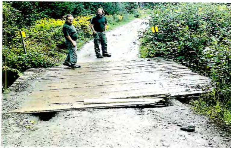
Figure 1, 2 and 3- Shows the broken boards on the bridges and the eroding approaches.
