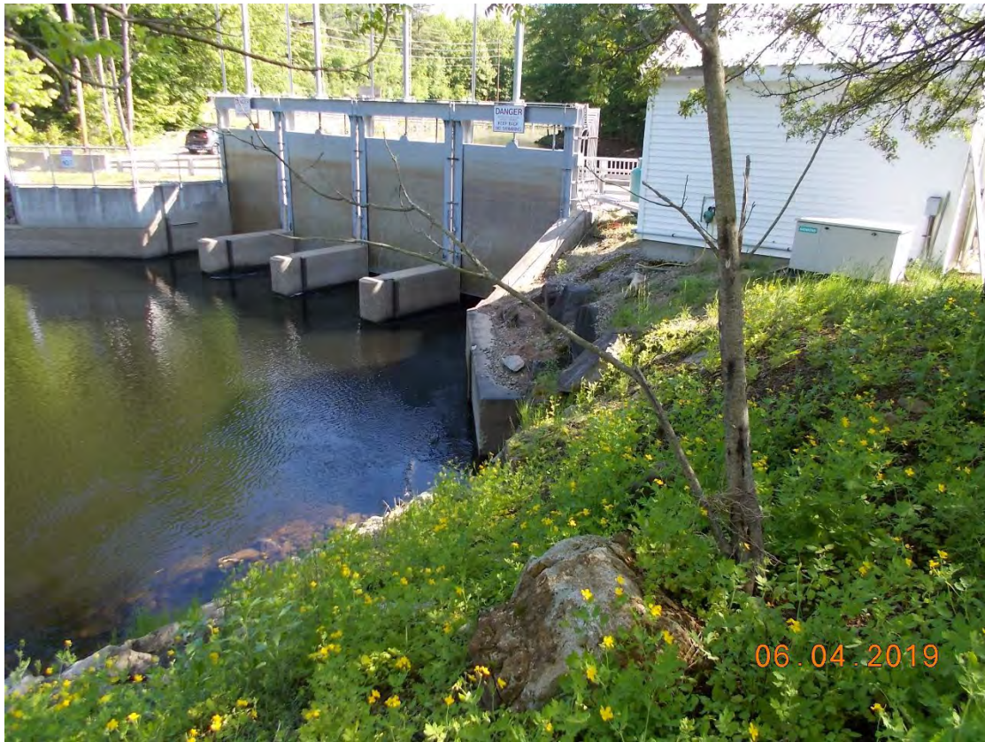
Figure 6. Rolfe Canal Gates
