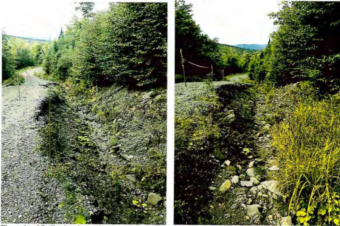
Figure 6 and 7- Depicts the washout along the trail.
