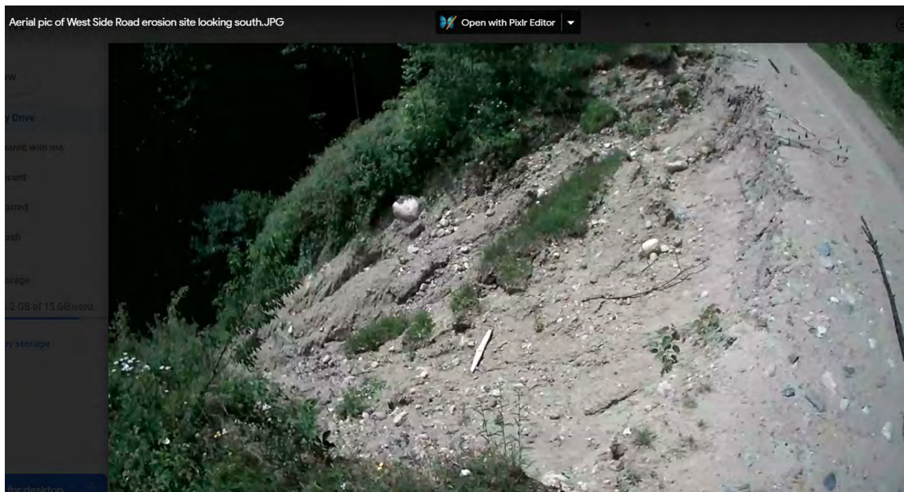
“Aerial pic of West Side Road erosion site looking south” (Board of Trails files.)
