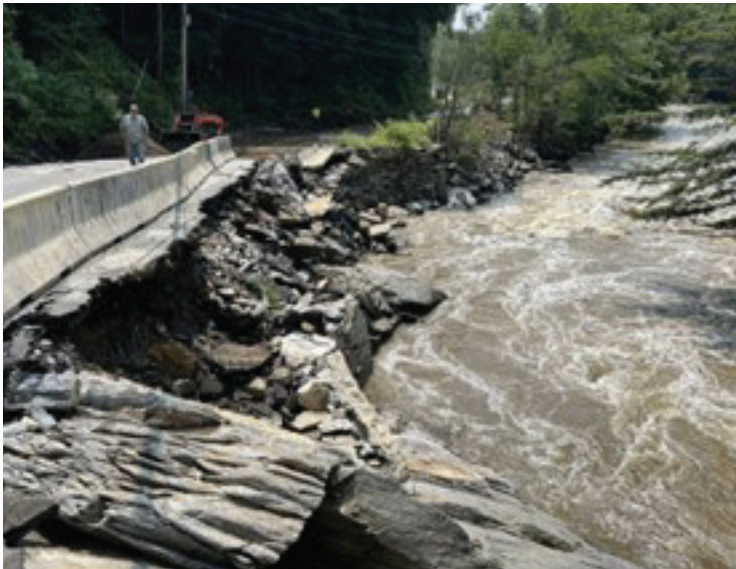
Flooding along Route 123A, Alstead, NH, July 2023
