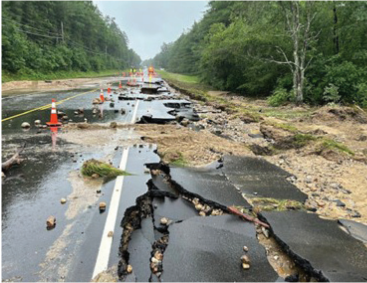
Flood along Route 10, Winchester, NH, July 2023
