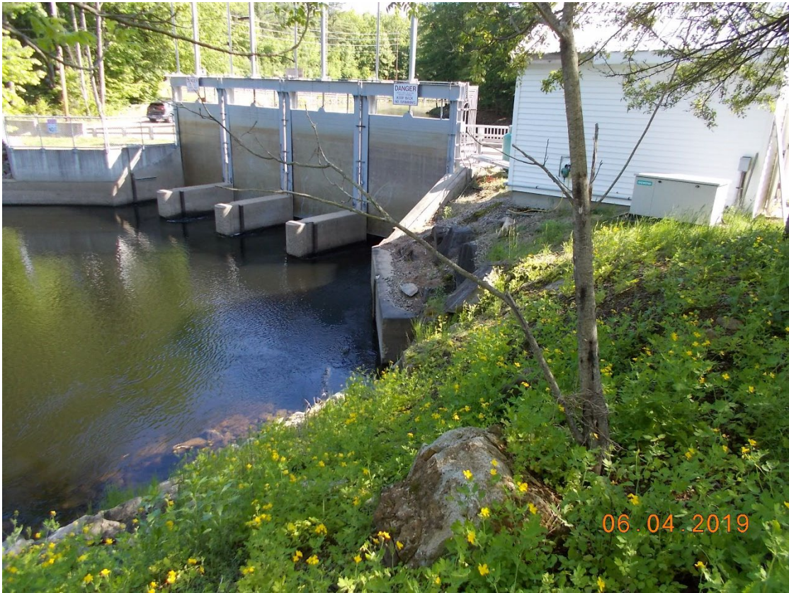
Figure 6. Rolfe Canal Gates
