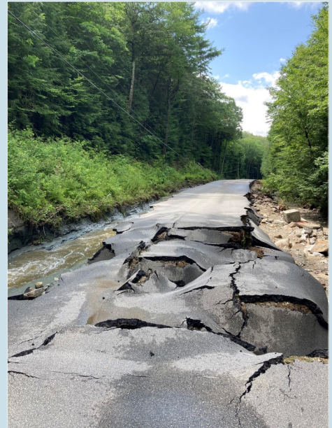
Road damage in Acworth (Source: NH Electric Cooperative)
