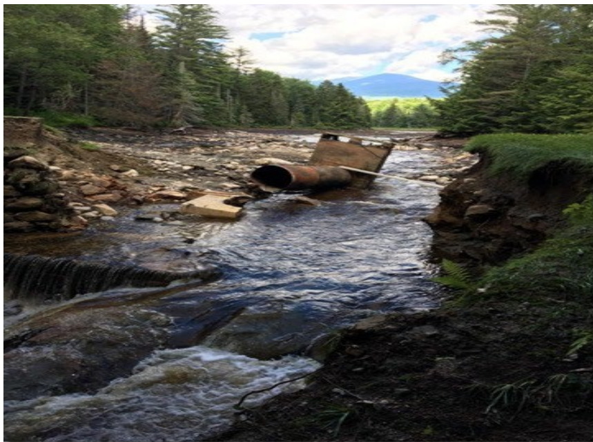
Photo 2: Looking northeast at failed Weeks dam and washed-out Gould Hill Road in 7/2017.
