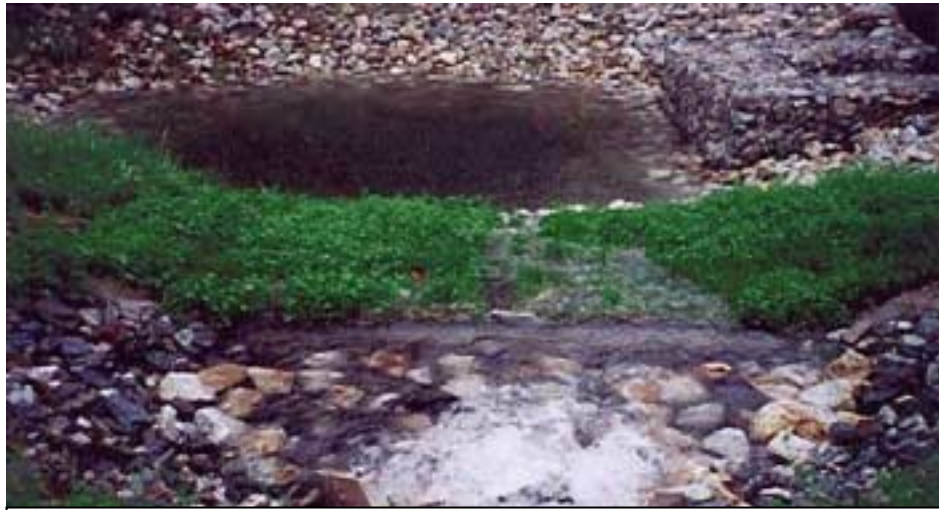
This pretreatment basin or sediment forebay has simple construction using a gabion (rock filled wire basket) berm. This helps reduce the velocity of the flows and settle out some sediments before the water is treated further.
