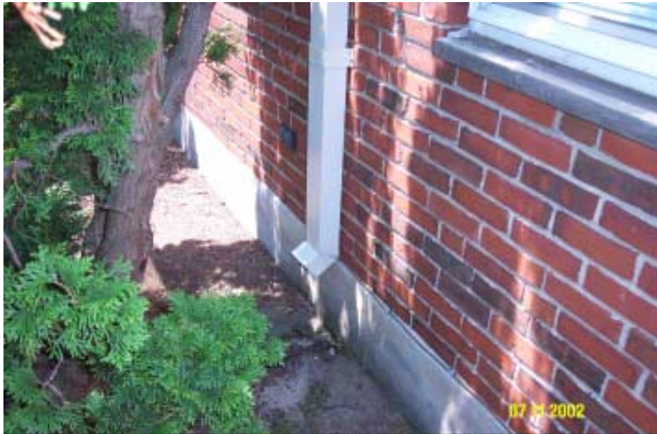
This roof leader from a large apartment building discharges to a concrete pad and then to the street. It could easily be rerouted to the lawn area or a drywell set several feet from the building.
