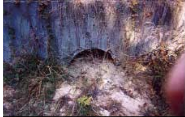
This drainage pipe, located in a subwatershed of Pennichuck Brook, shows evidence of the high volume of sand and silts that enter this waterway via stormwater.
